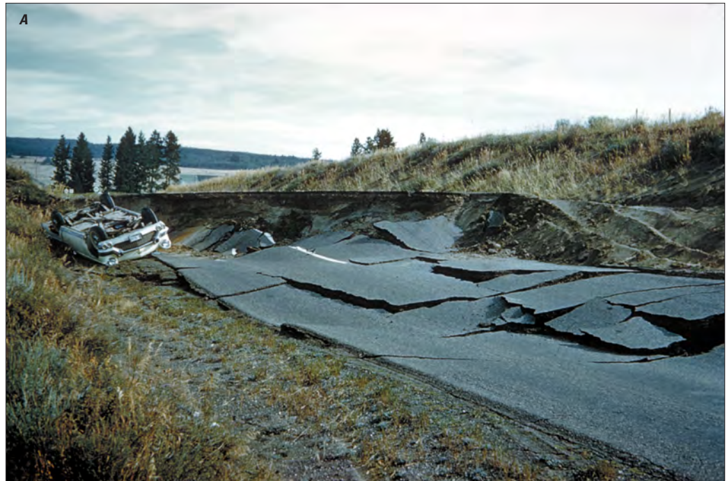
Figure 5. Photographs showing examples of types of damage to lifelines and infrastructure expected to occur along the Hayward Fault in the San Francisco Bay region, California, in an earthquake like the magnitude-7 mainshock modeled in the HayWired scenario. A , Damage to a road from fault offset; B , column of water gushing from a damaged pipeline; and C , large electrical conduit broken by fault offset. (Photographs from National Information Service for Earthquake Engineering-Pacific Earthquake Engineering Research Center (NISEE-PEER), University of California, Berkeley, used with permission.)
