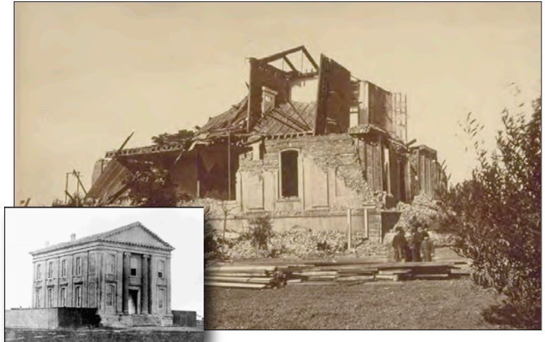
Figure 3. Photograph showing shaking damage from the 1868 magnitude-6.8 Hayward Fault earthquake, which caused collapse of the Alameda County Courthouse in San Leandro, California (photograph courtesy of the Bancroft Library, University of California, Berkeley). Inset shows the same building before the earthquake (photograph courtesy of San Leandro Public Library).
