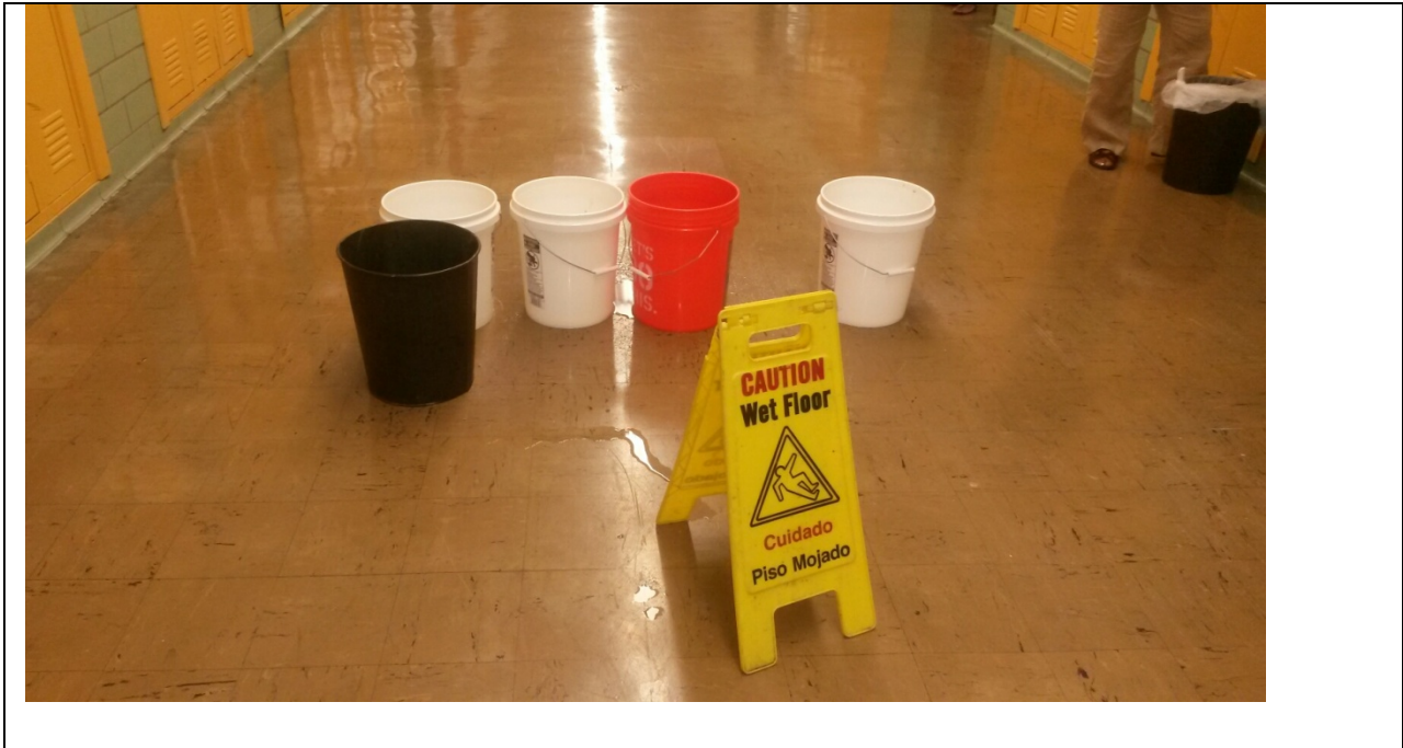
Figure 15: Buckets Collecting Leaks in the Hallway at Cody MCH, August 2016
